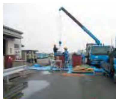
Machinery containing PCBs being shipped to treatment site
