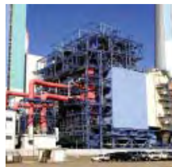
Dry-type flue-gas desulfurization system at Isogo Thermal Power Station's new No. 1 unit.
