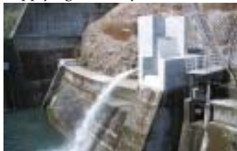
Sufficient water to maintain river levels is released from the spillway (Taio Mini Hydropower Station, Oita Prefecture)
