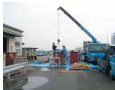
Machinery containing PCBs being shipped to treatment site (Wakamatsu Operations & General Management Office, Fukuoka Prefecture)
