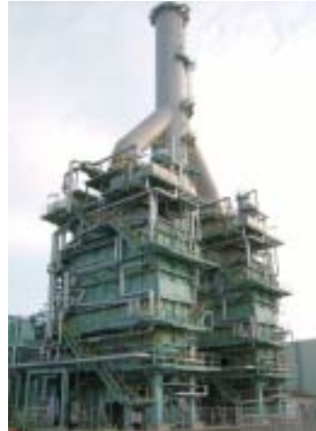
Ichihara Power Station (Chiba Prefecture)
