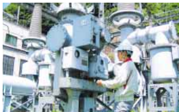
Inspection of gas pressure of switches (Sakuma Power Station)
