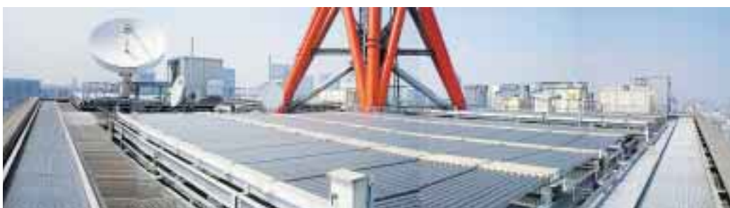
Solar panel for indoor hot-water supply (on the roof of the head office building)
