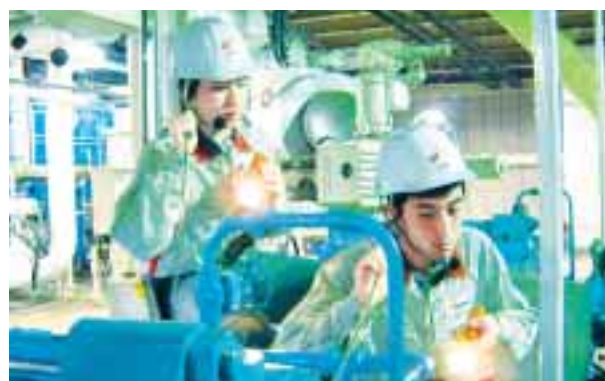
Audible inspection of pumps (Isogo Thermal Power Station)
