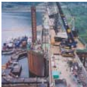
Introduction of new technology at our Okutadami Power Station made it possible to increase the facility's capacity to 200 megawatts without changing the water level.
