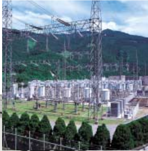
Sakuma Frequency Converter Station
