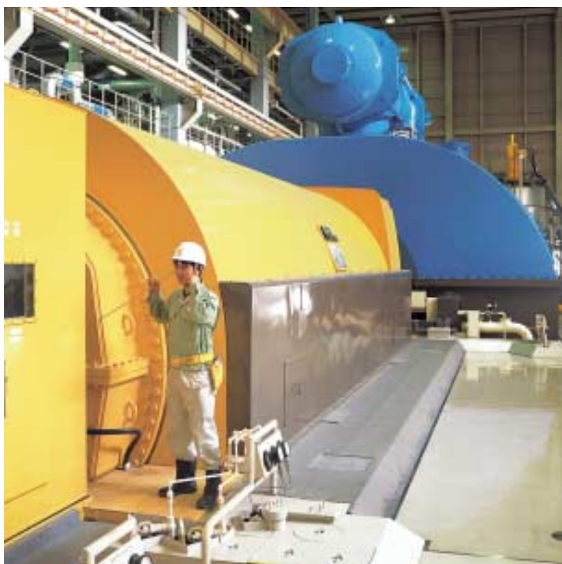
◀ Isogo Thermal Power Station
